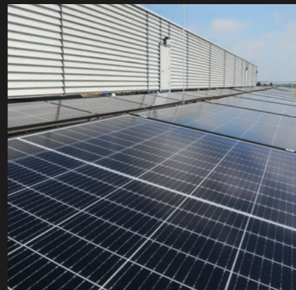
Rooftop solar PV scheduled end of 2022
