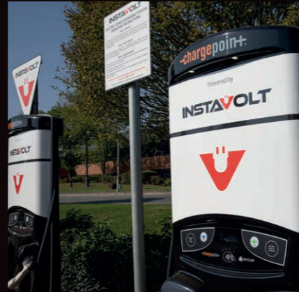
Electric vehicle charging
