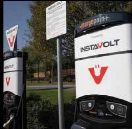
Electric vehicle charging
