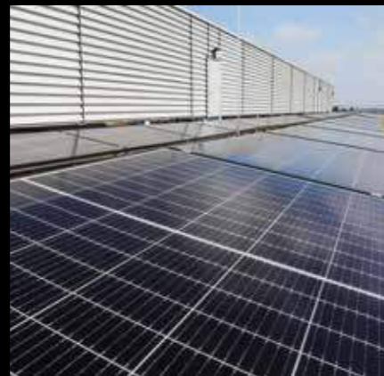
Rooftop solar PV
